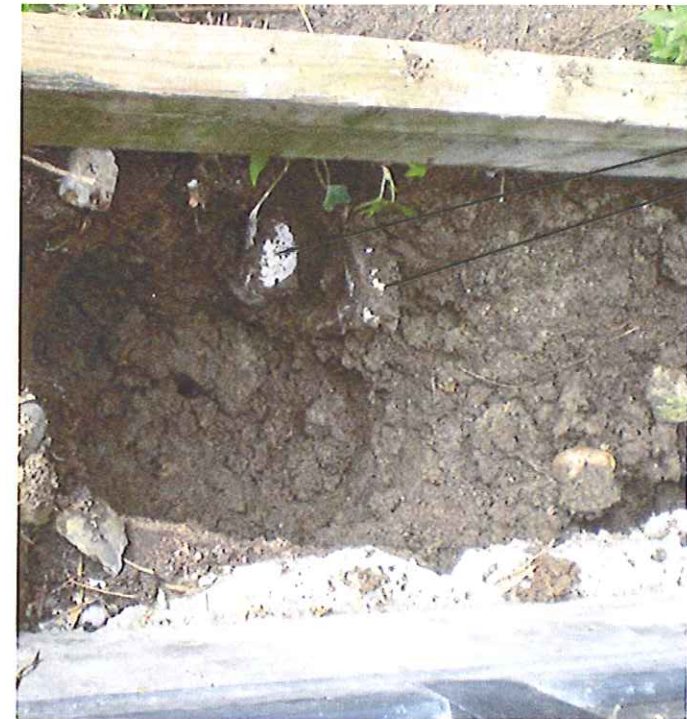
PHOTO 1 NEW PW CONNECTION TO POND FEED LINE
